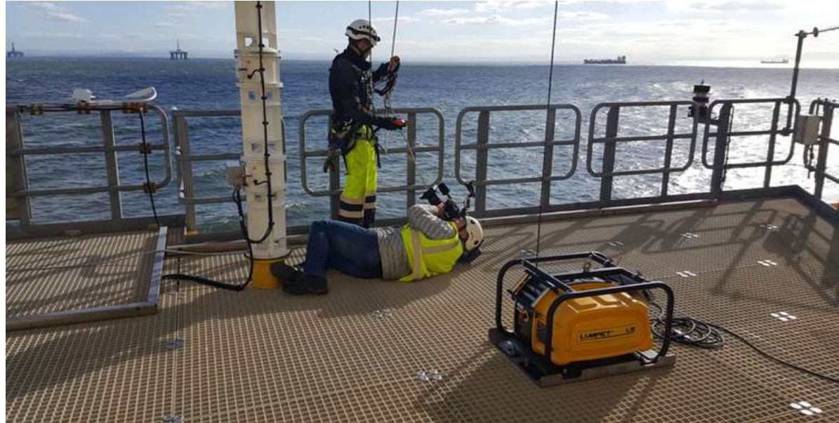
Limpet Technology Demonstration
